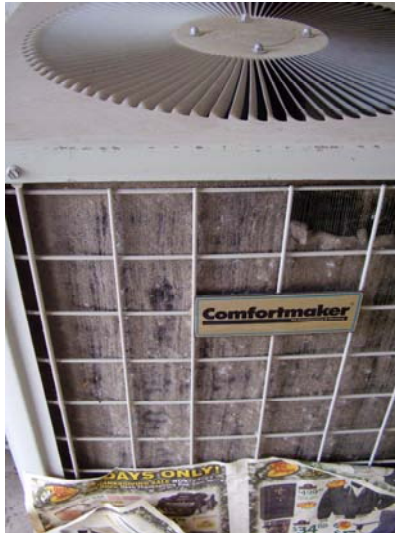
(not only are the coils coated with cottonwood – newspapers are also blocking part of this unit)
