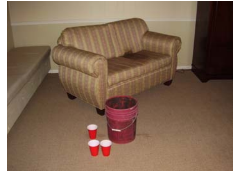
(water leaks have badly stained a couch and fill buckets and cups)
