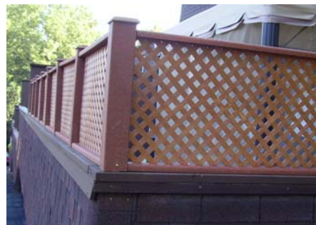
(new privacy screen installed according to condo guidelines regarding size and color – approved by board)
